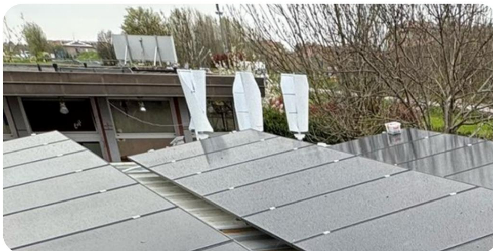
INSTALLATION OF 3 2KW TURBINES COMBINED WITH A SYSTEM 12KW PHOTOVOLTIC SYSTEM IN A PIZZERIA IN BOLOGNA
