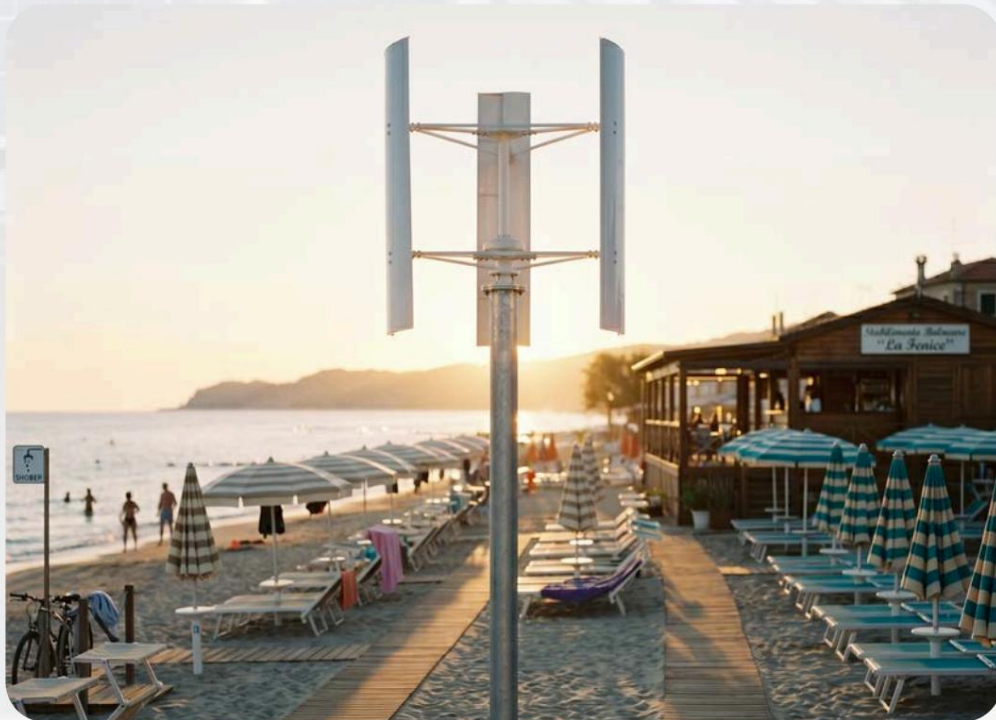
INSTALLATION OF AN H-TYPE TURBINE IN A SEASIDE RESORT
