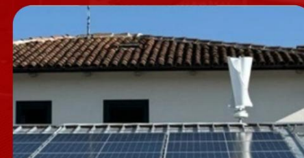
HYBRID WIND PHOTOENERGY INSTALLATION
